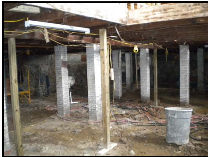
Basement view of former brick vault location (note ceiling open to first floor).
