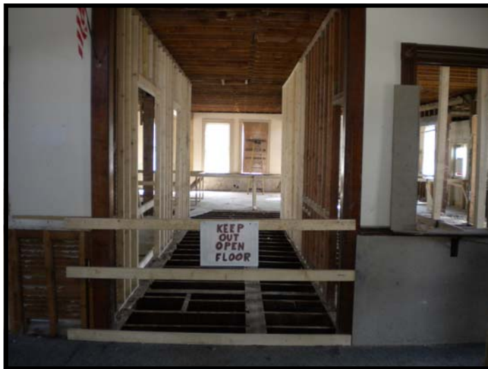
View of 1st floor hallway. (Area with flooring removed is approximate area of new staircase down to the ground level.)
