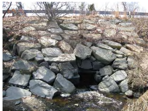
Figure 3-27. Damon's Point Dam downstream spillway.
