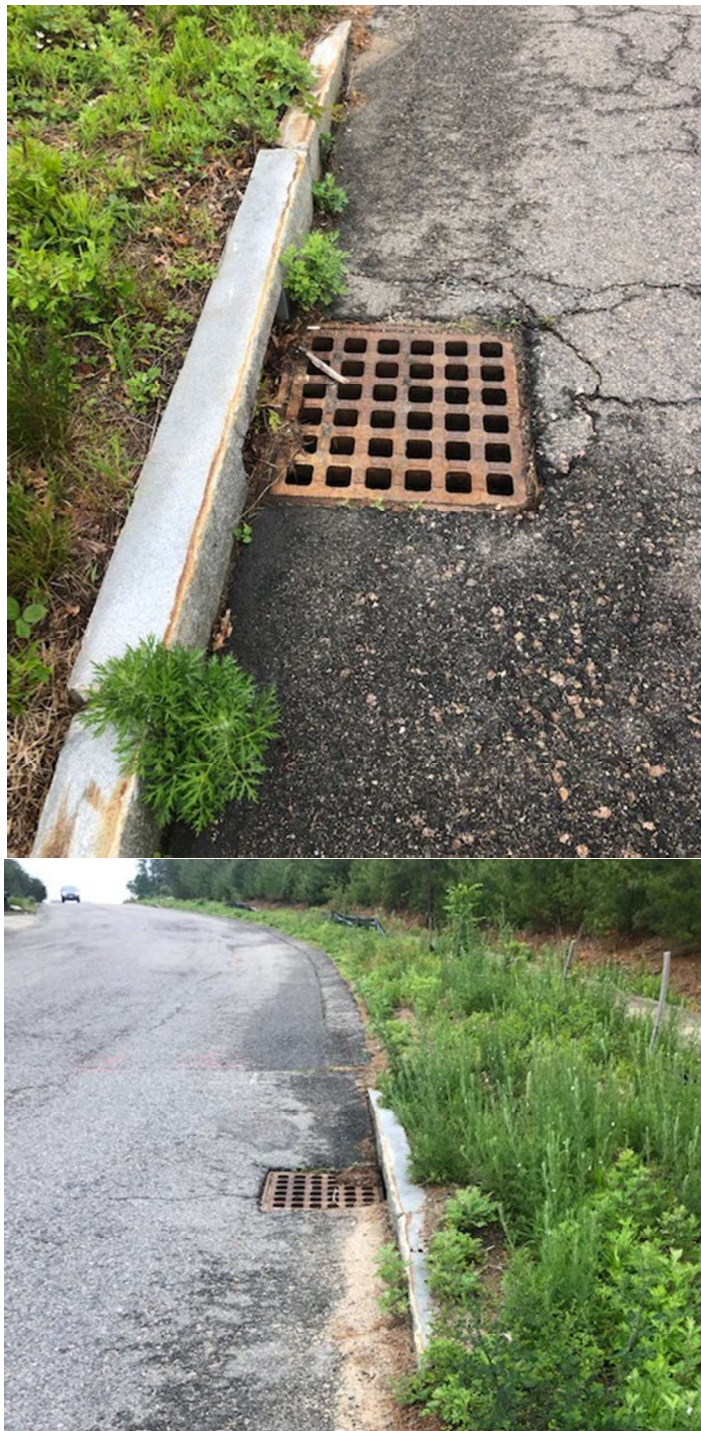
Commerce Way Catch Basins
